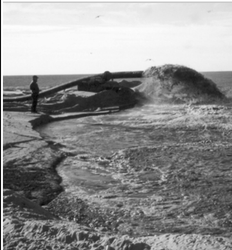
Dredge spoils are pumped through the pipe and deposited on the island
