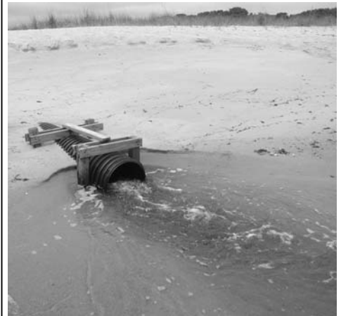
Partially buried exchange pipe between Nantucket Sound and Rushy Marsh Pond Summer 2005
