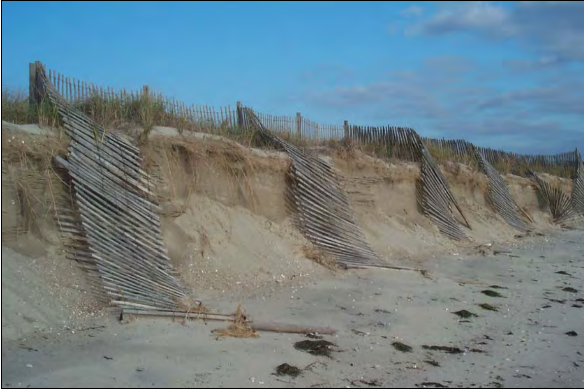
Figure 2. At the time of the November 2002 shoreline survey of Dead Neck, sand fencing set-up in the nourishment area had begun to fail due to erosion of the beach fill.
